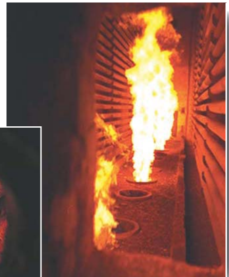
Gas Burner in Fire Box
