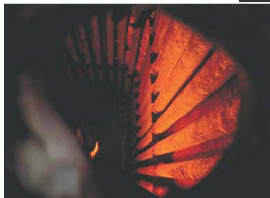
Fired Heater Tubes
